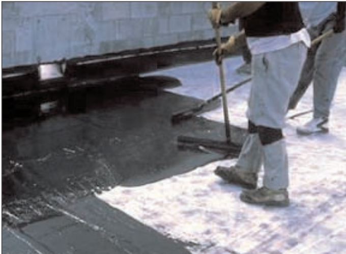
STRATASEAL HR reinforced membrane being installed over a concrete deck to a 215-mil (5.5mm) thickness.
